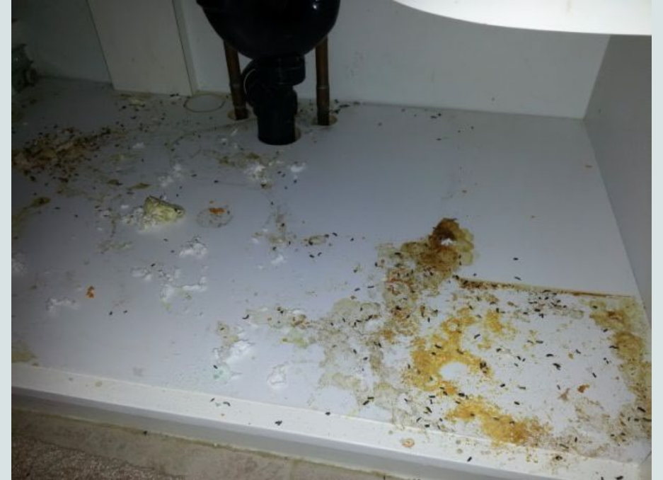
Mouse droppings and urine under a bathroom sink
